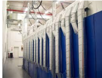
Battery Room Ventilation
